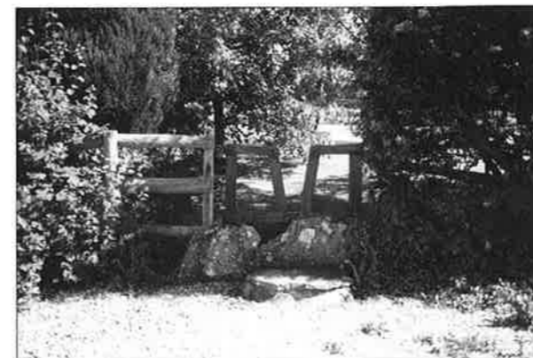
Fig 9: Delapidated stone stile and modern wooden stile on footpath
